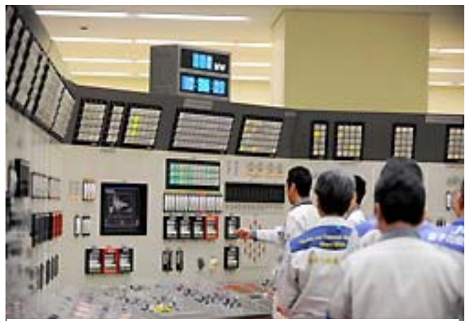
Fig.1 Inspection view at MONJU control room
